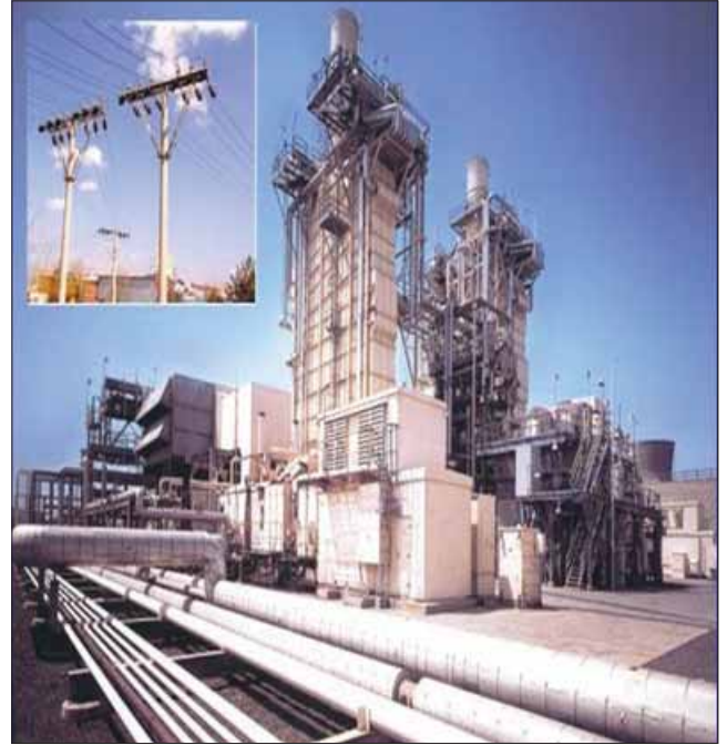
Natural Gas Power Plant in OSTİM Industrial Center
