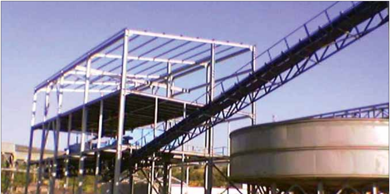
Coal washing and packaging plant in Bursa
